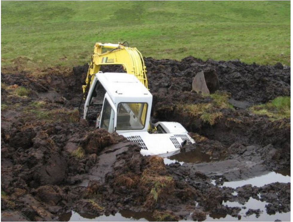
An excavator that is in a hole, and per the Law of Holes, has stopped digging.
